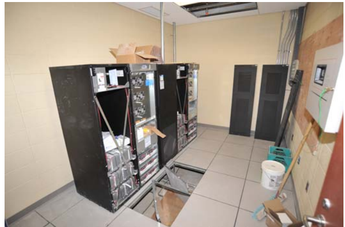
SPECIAL DESIGNED COMPUTER SERVER ROOM
