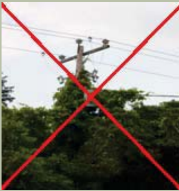
OVERGROWN VINES AROUND ELECTRICAL EQUIPMENT
