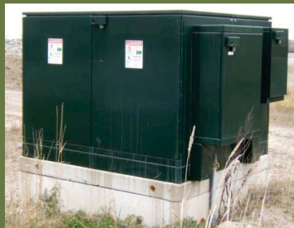
Pad mounted switchgear
