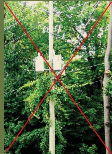
Pole growth contacting electrical equipment & powerlines
