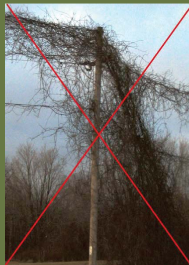
Guy-wire growth contacting electrical equipment & powerlines
