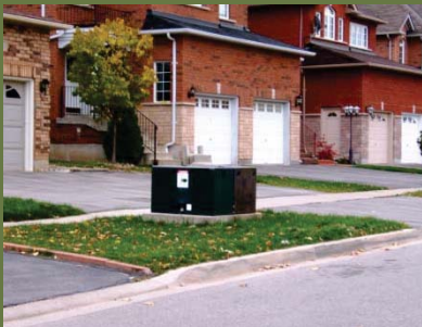
Pad mounted transformer
