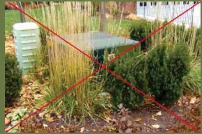
Obstruction around a transformer
